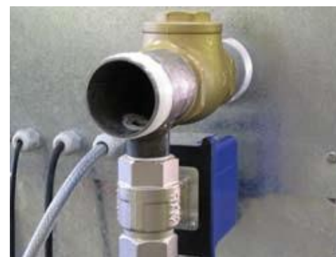
Auto line drain.
